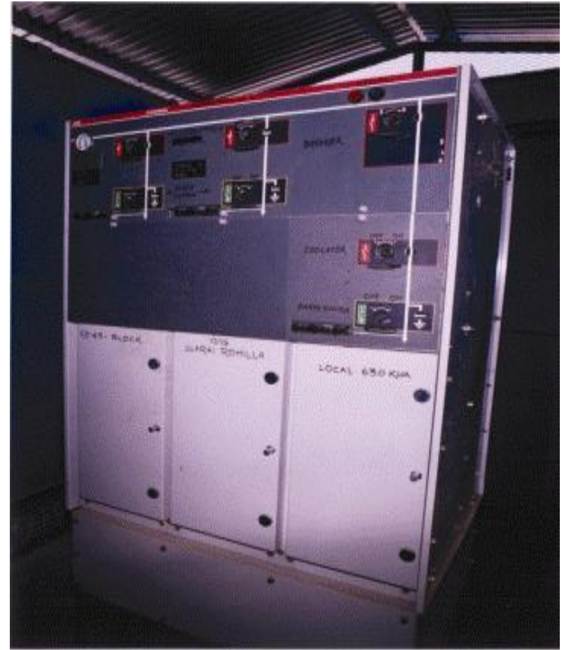
After : New Ring Main Units
