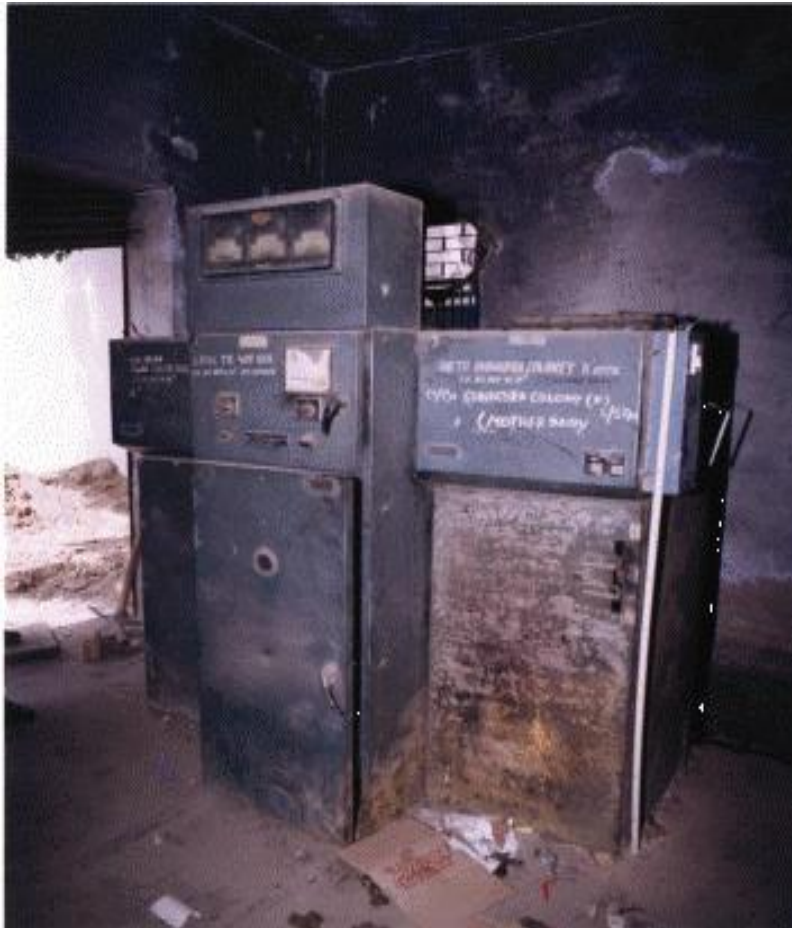
Before : Old Switch Gears
