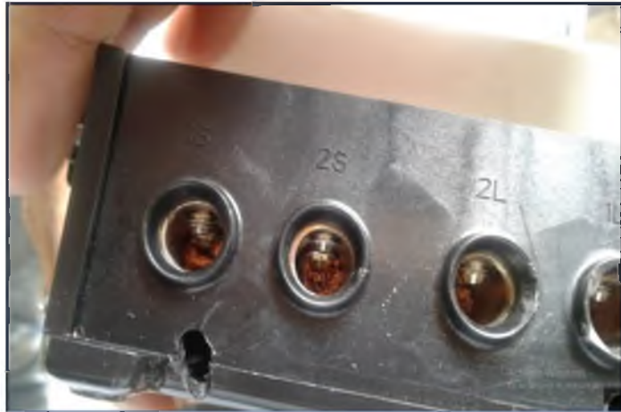
1) Shunt Found in Meter Terminal
