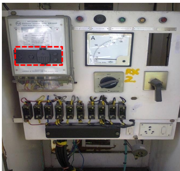
Defective meter at FI Smith S/S in Vellore Circle
