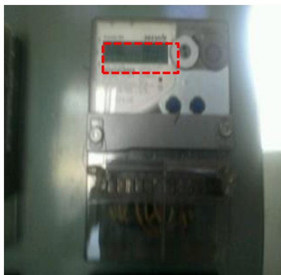
Defective meter in Erode Urban division in Erode circle
