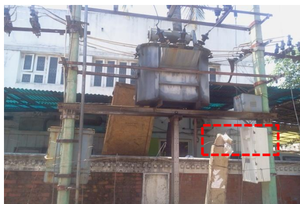
Defective DT meter installed in Samayanallur division in Madurai
