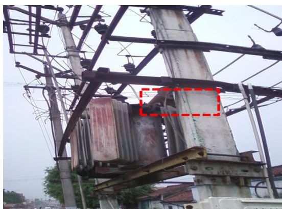
No. meter installed in the DT located in the ARCOT division of Vellore
